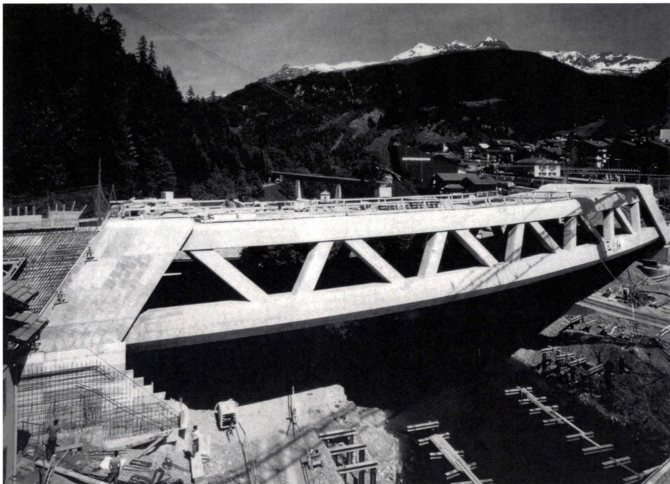
Gesamtansicht der Landquartbrücke general view of the bridge over the Landquart river
