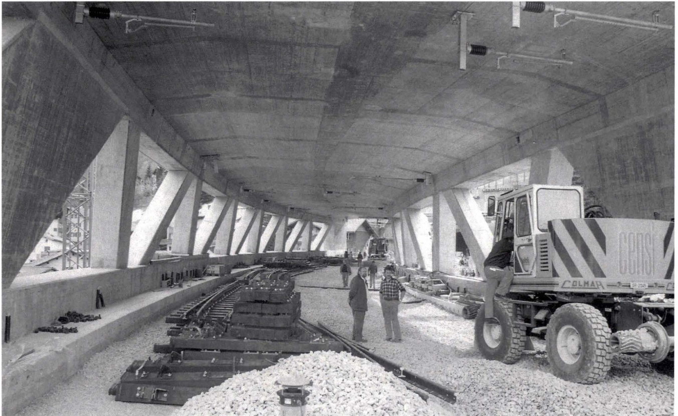
Blick ins Brückeninnere, Vorbereitung des Geleisebaus Interior view with preparation of the two tracks
