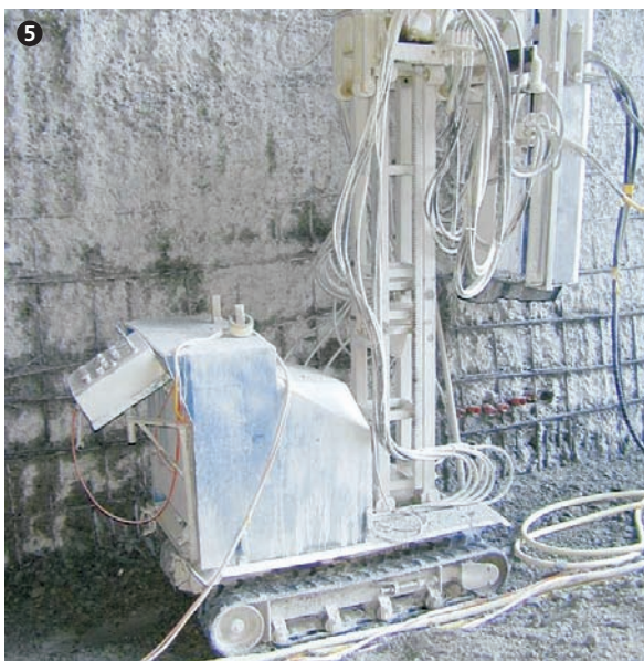
5 HDW-Roboter. High-pressure water robot.
