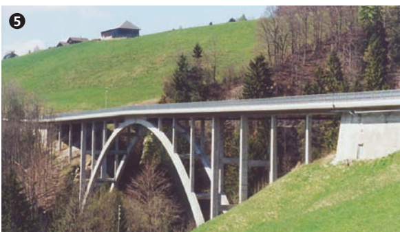
5 Pont sur le Javroz après l'intervention. General view of the bridge after the intervention.
