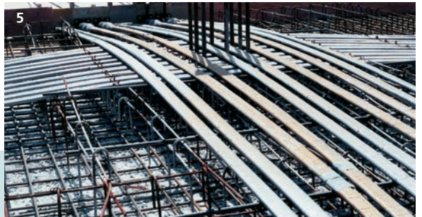
10 herkömmliche Spannglieder, angeordnet in Stützstreifen. 10 conventional post-tensioning tendons, placed in support strip.
